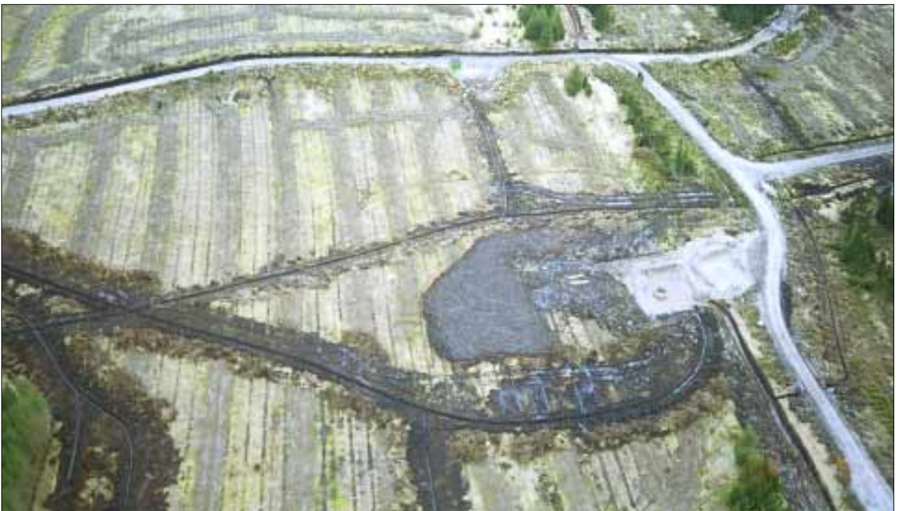
Plate 6: An aerial view of the site showing floating roads used for access tracks and a near-complete turbine base awaiting final mineral back-fill. Note the excavated peat side-cast and left exposed. The light green/grey areas are trees cut by a 20-tonne tree harvesting machine and laid in rows to support the weight of the machine as it progresses on the blanket bog. The trees have been left to decay.
