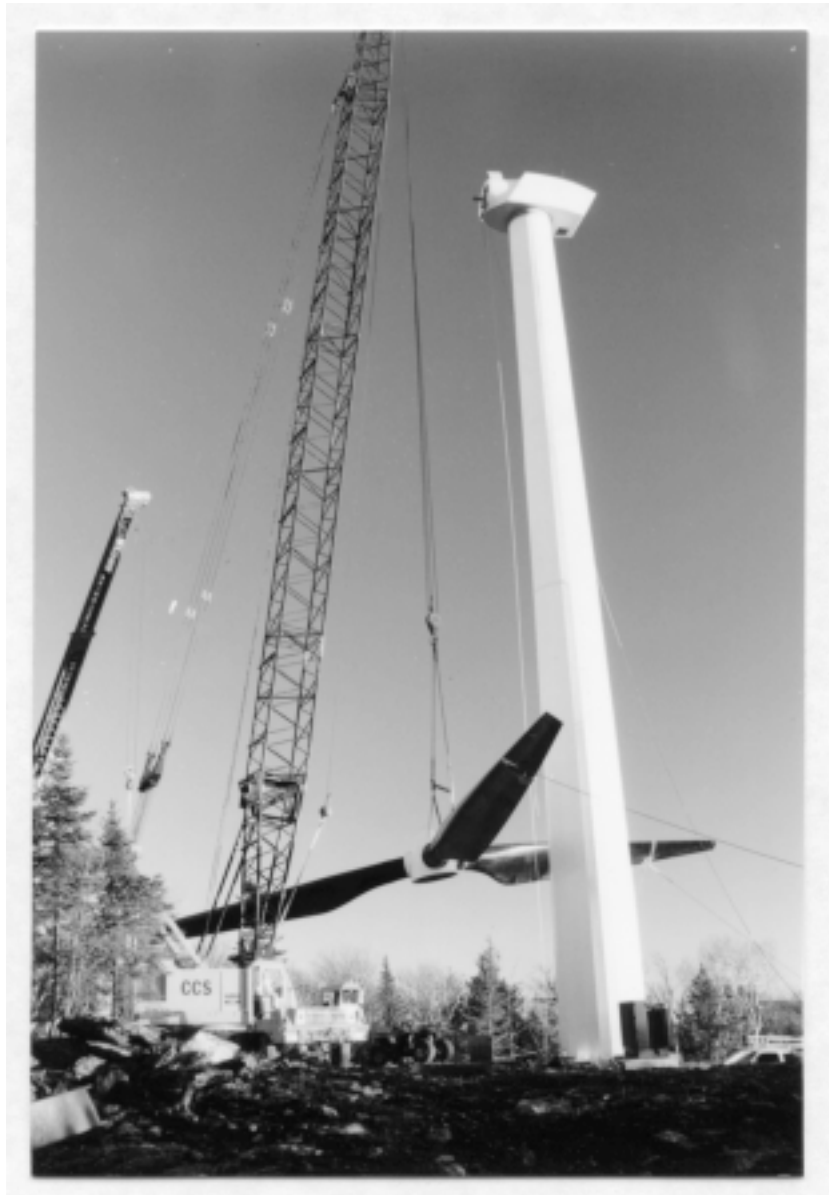
Figure 6-6 Lifting the Rotor Assembly for Attachment to the Nacelle. Note the limited area for lay-down purposes.
