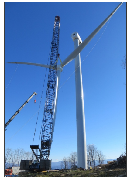
The first rotor is hoisted in to position at Site #2 on a crisp, clear November 14th.
