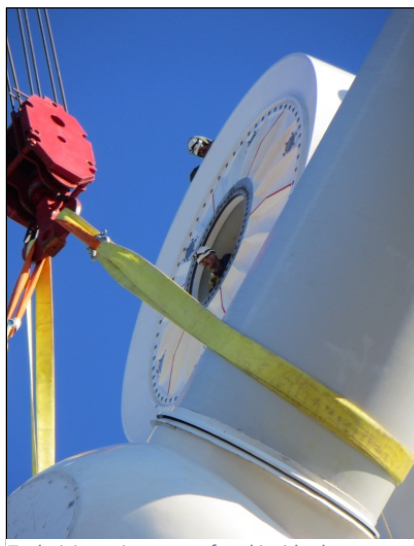
Technicians sit on top of and inside the generator guiding the rotor as it is lifted into position.
