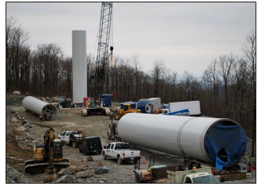
Large turbine parts arrive for assembly make for a busy construction site in early November.
