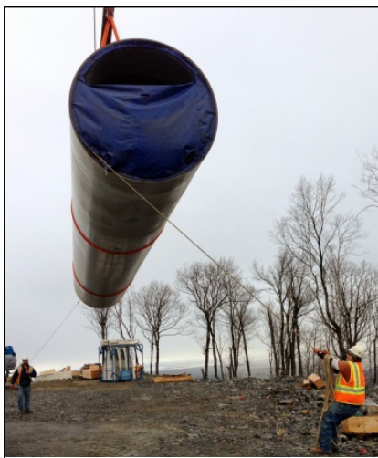
A construction worker guides the offloading of a tower section near the turbine pad.
