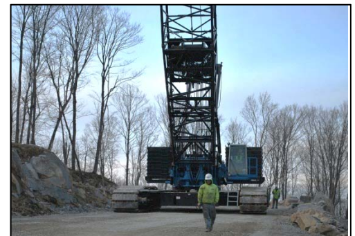
The Manitowac 16000 crane, with its 31’ track crawls to the next wind turbine pad site.
