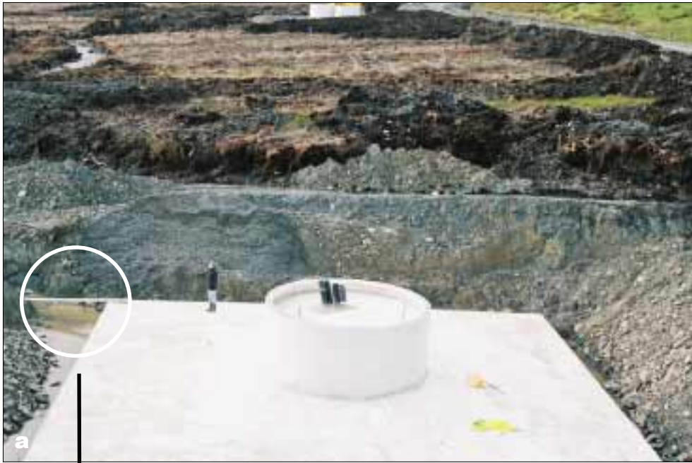
Plate 14a: the excavation for base 28. Even if this is back-filled with 'borrowed' mineral, the adjacent peat will dry out and oxidise over time. The drain runs into a waterway visible in the top left of the picture. b: the view down the channel draining turbine 25.
