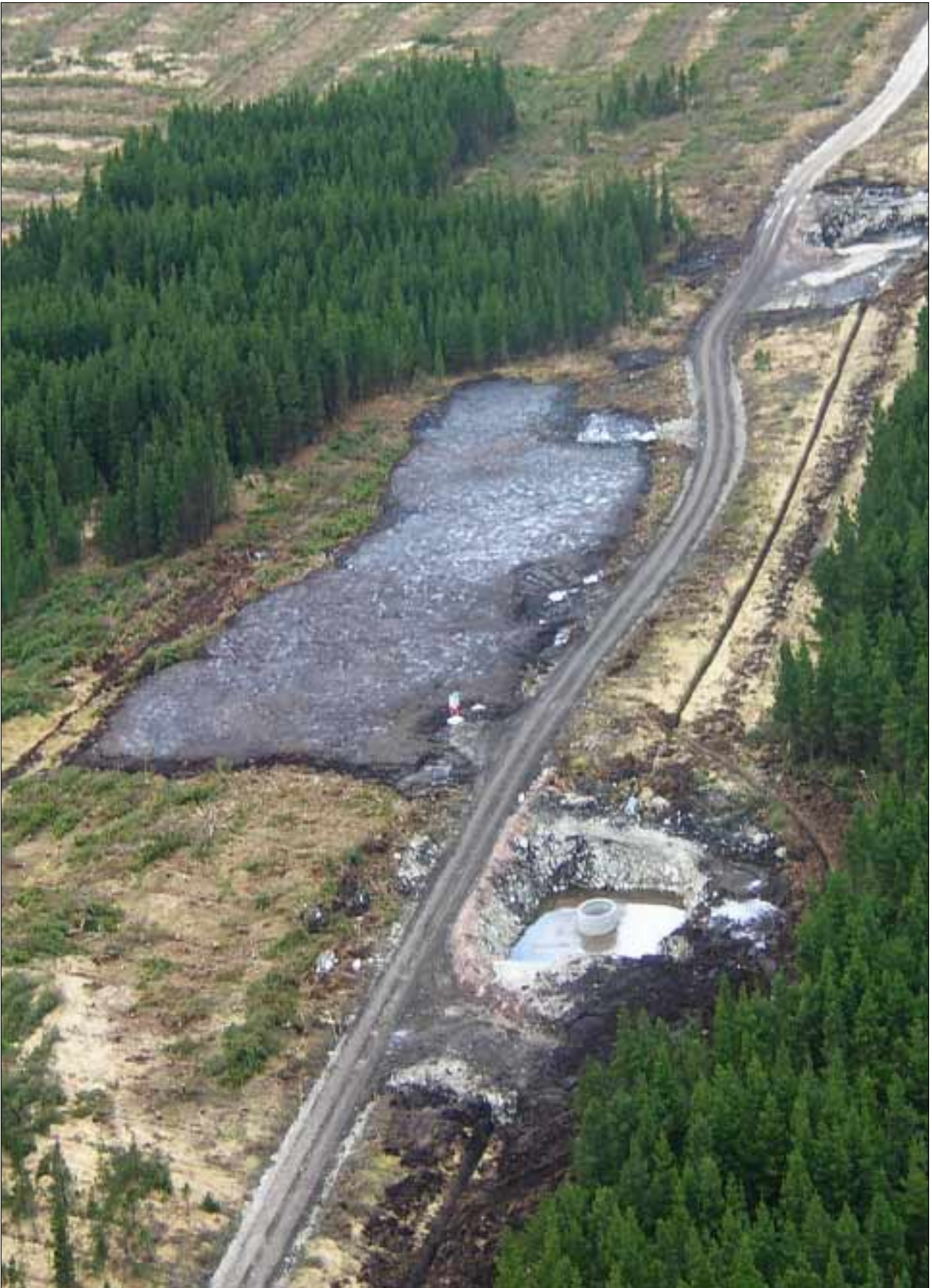
Plate 8: two turbine bases at Derrybrien (middle foreground and top right) awaiting mineral backfill. Note the ‘floating’ access track, mineral-filled drainage, cable trenches and extracted peat laid on top of intact blanket bog, where it will dry out and oxidise over time. The remaining conifers have since been felled.
