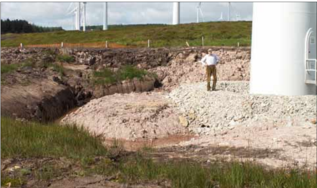
Plate 23: A completed turbine base on Derrybrien showing exposed peat which will oxidise and erode over time. While other peatland projects propose different construction techniques, the risk of pollution and landslip remains whenever such terrain is industrialised, whatever the perceived political acceptability of its purpose.
