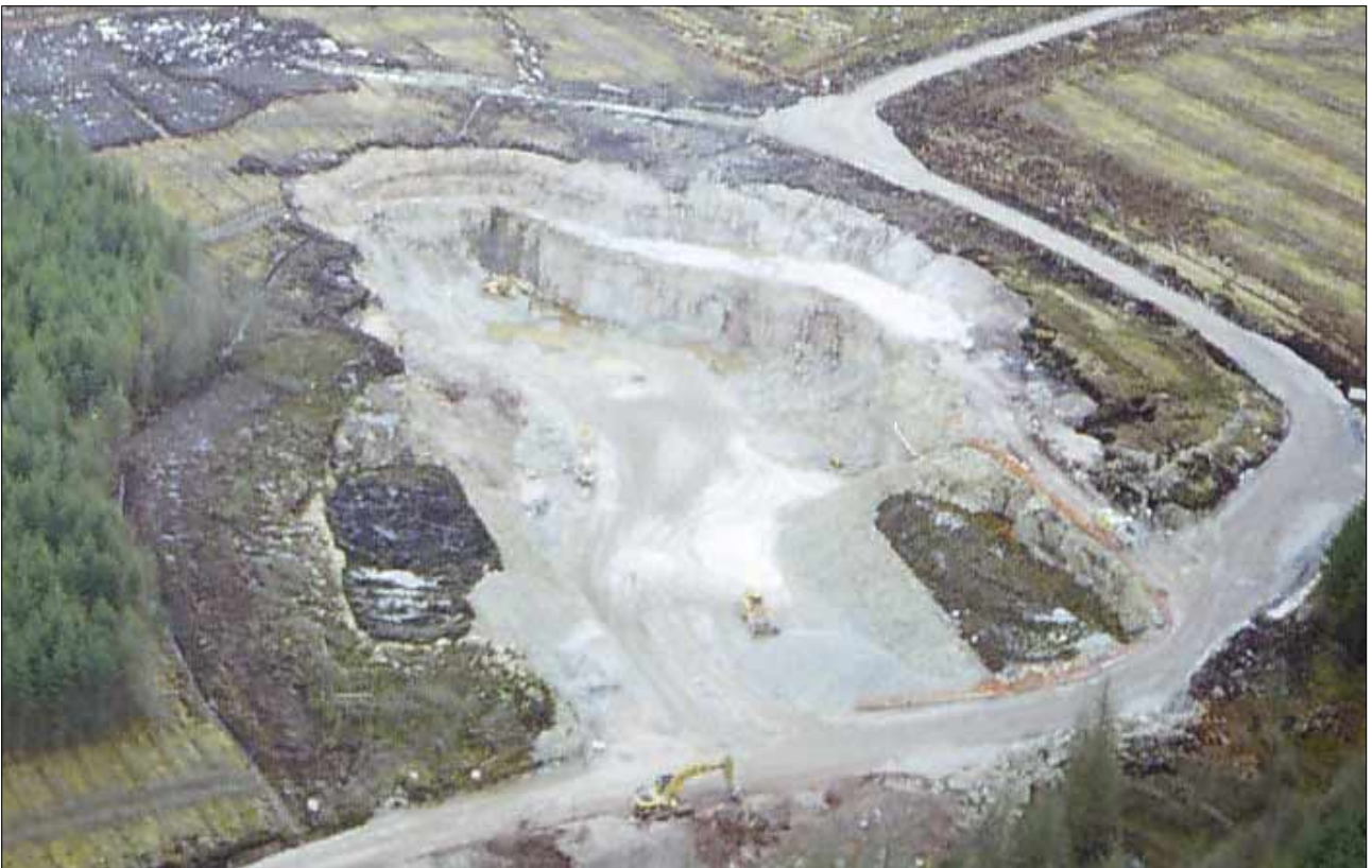
Plate 8: An aerial view taken in April 2005 of the largest 'borrow' pit on the site, excavated from stratified limestone and originally over-burdened with two metres of peat and three of boulder clay, seen here cast to the side. The excavators suggest the scale. Its volume is estimated at 150,000 m 3 .
