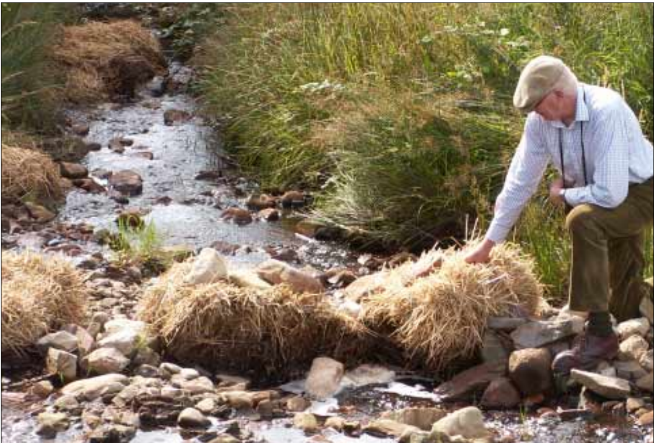
Plate 14: A ‘silt trap’, sited adjacent to the above lagoon, made from barley-straw bales. At low flow levels, the water runs through the stones in the stream bed and little, if any, of the suspended matter is trapped. When the flow is high, it pushes the bales aside and the increased load of suspended matter again goes straight down the watercourse. Two displaced bales can be seen on the top left of the picture. Unless these bales are replaced on an eight-week cycle, their decomposition is itself pollutant.
