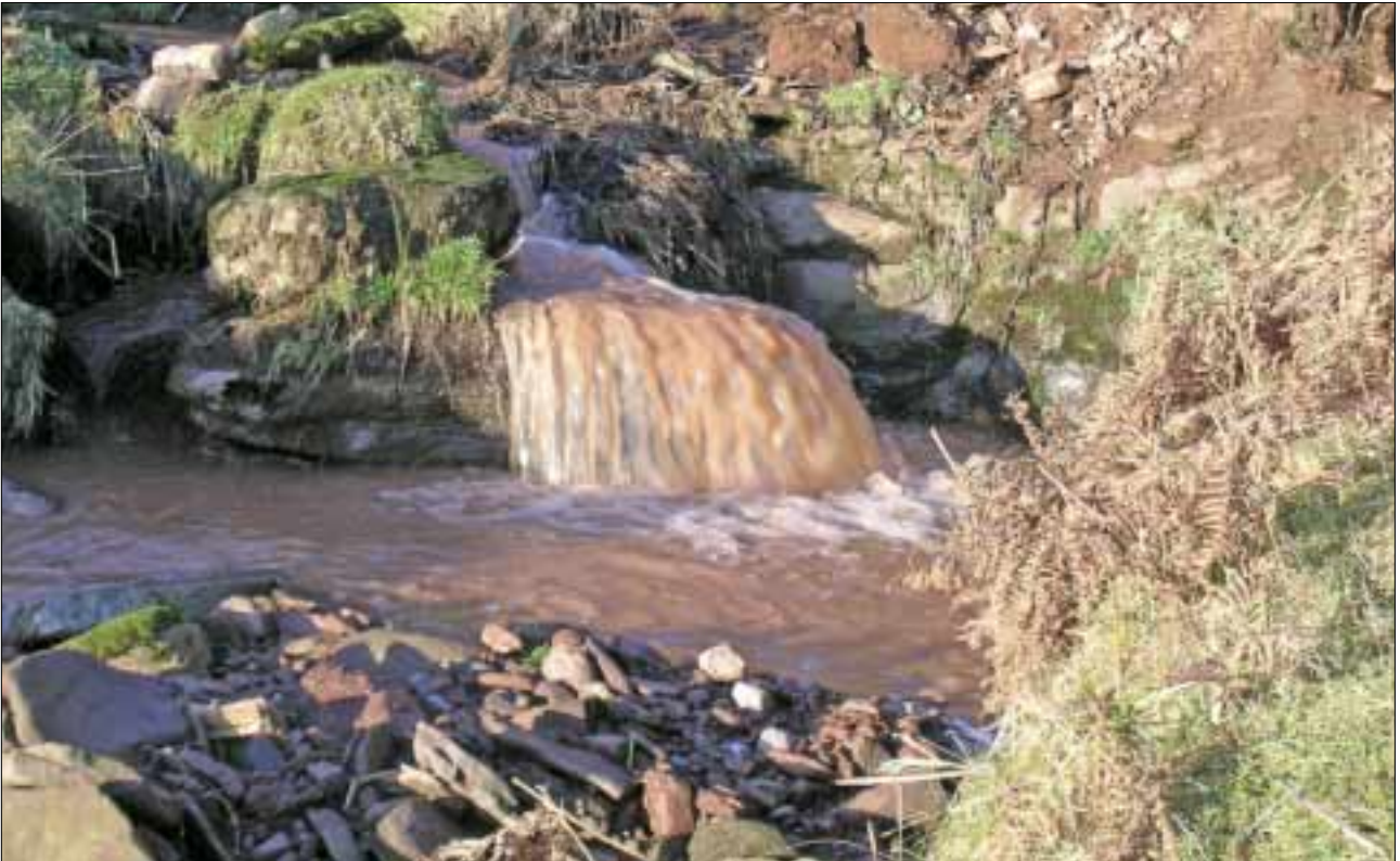
Water draining from a newly-constructed track road driven seven kilometres east of the Braes of Doune site to allow access to its grid connection. When this picture was taken, polluted run-off from the tracks was flowing unimpeded into local waterways before entering the Bullie Burn (above) and on into the River Teith Special Area of Conservation. (12 December 2005, NN 813 104.)
