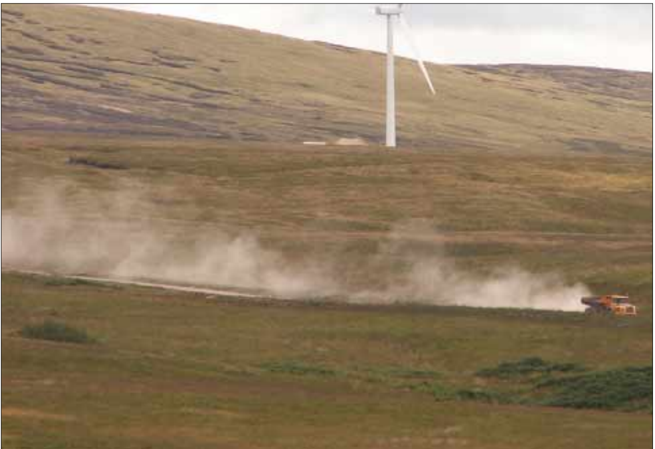
Site traffic, which passes nearby constantly, suggests the quantity of material that will eventually be washed down the local waterways.
