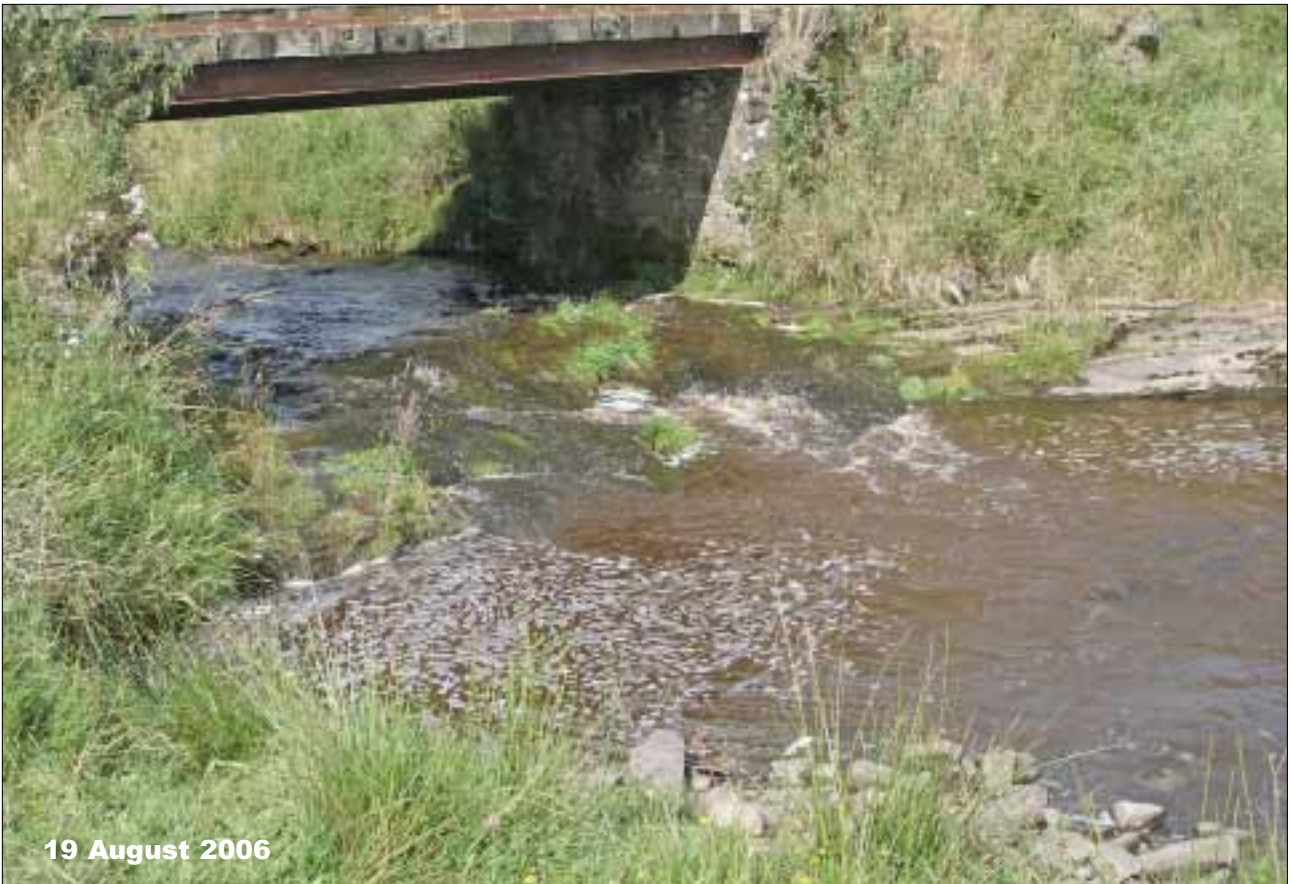
The Severie Bridge (cf page 21) seen here on 19 August, a week after the picture on page 22. Despite only light precedent rainfall, the burn is clearly loaded with silt.
