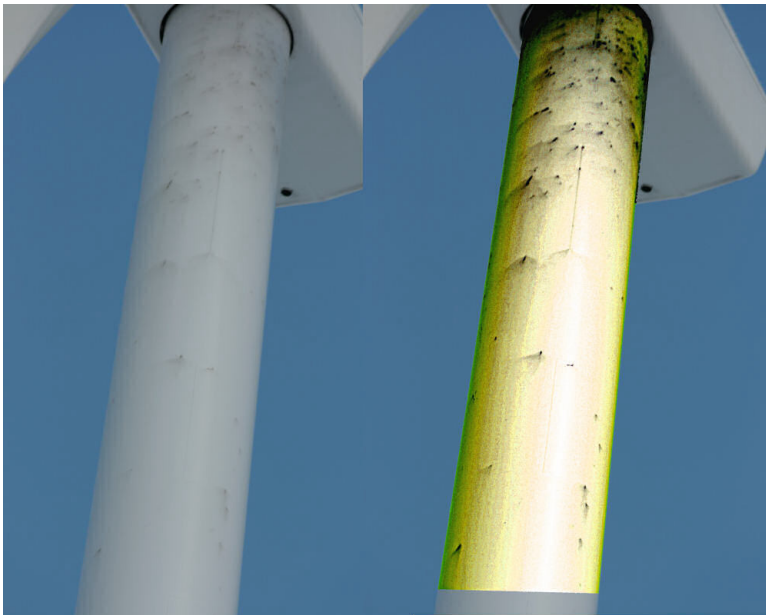
Richmond Road turbine, March 1 st 2008 Image enhancement used to clarify the spatters
